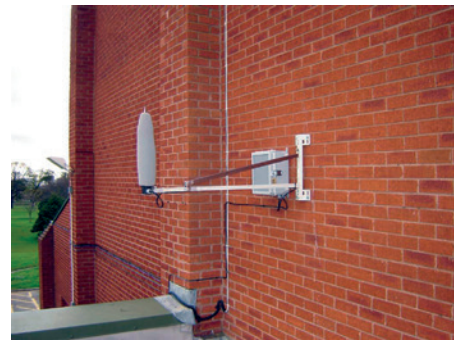
Figure 4: Example of a customized long term noise monitoring system for monitoring of offshore construction noise
