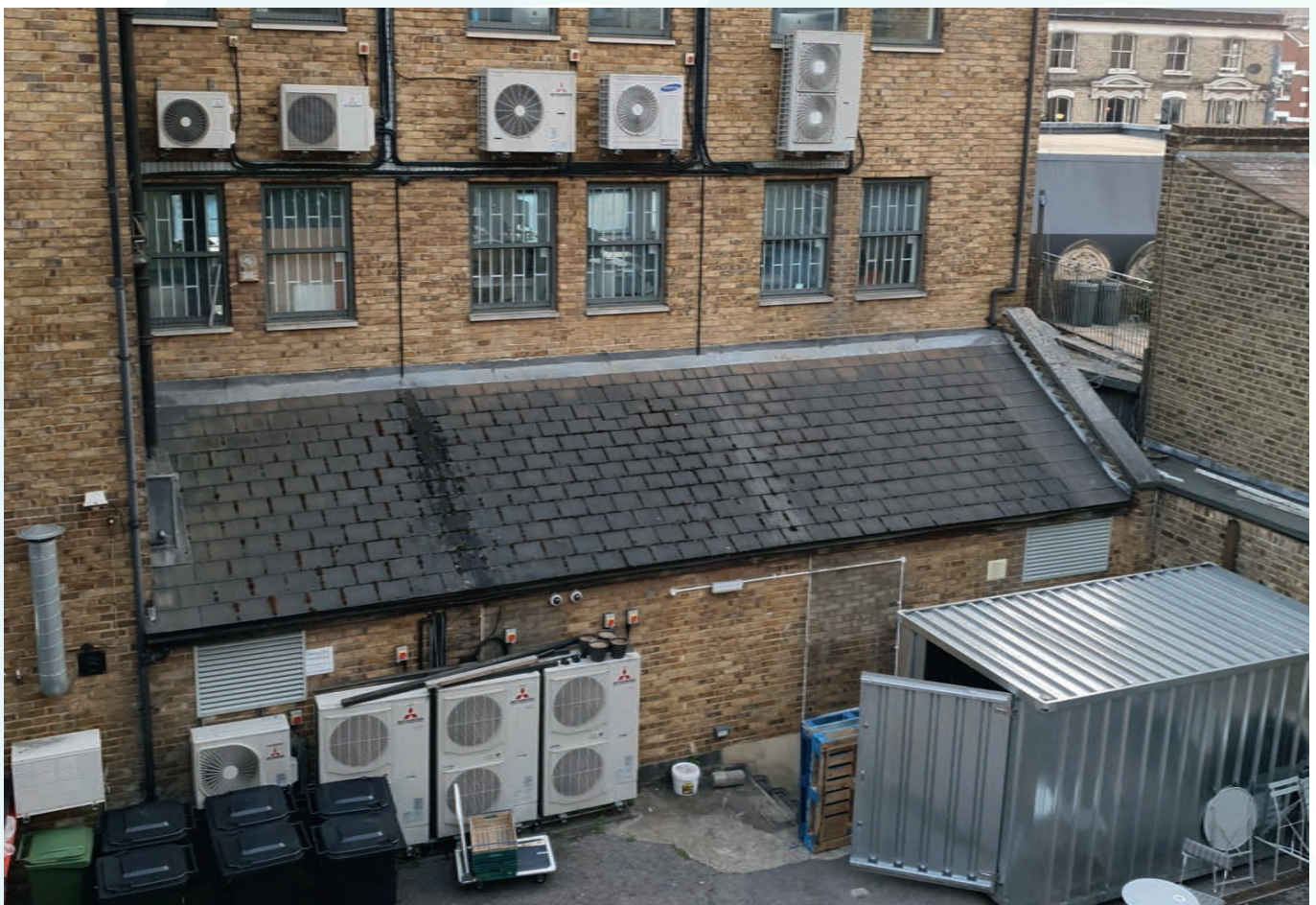
Below: Urban location with multiple existing AC units
