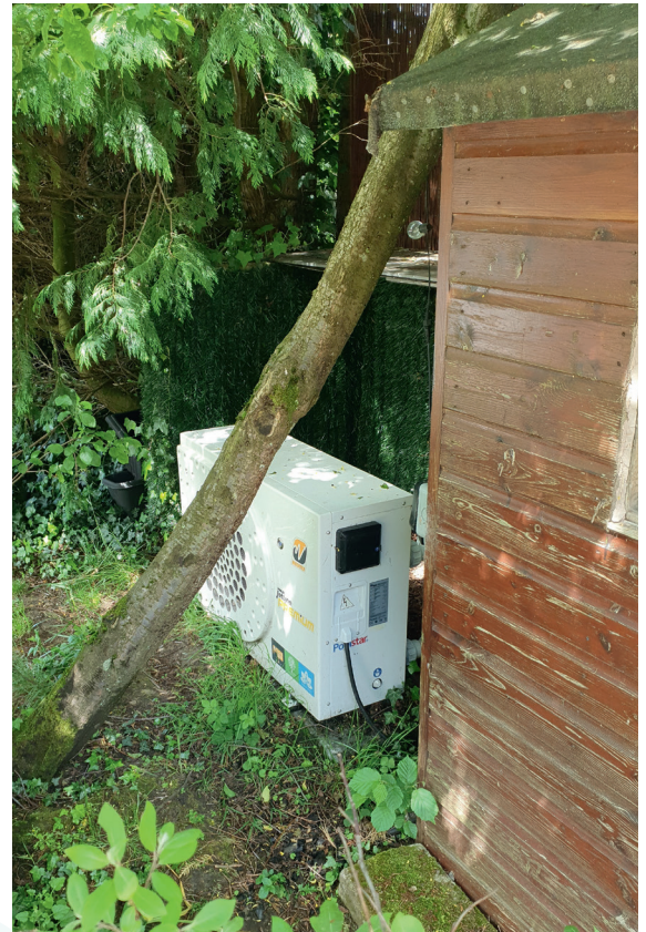
Above: Air source heat pump in a garden
