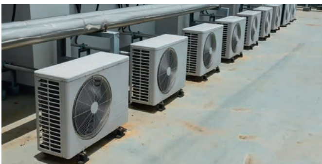
Above: The most recent Midlands Branch meeting focused on of vibration isolation of heat pumps and HVAC
