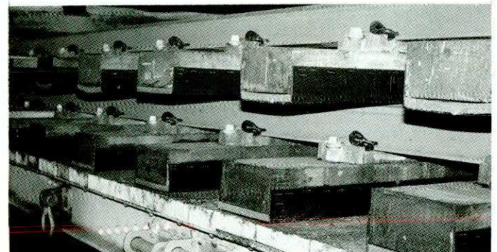
Fig. 7. Under-sleeper isolators stacked.
